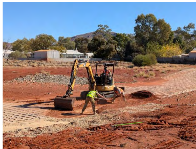
Image 2 – CPL Volta, SPR Bell and SPR Carbone battle the flies whilst conducting defects rectification works on the Flood Management System in Amata.
