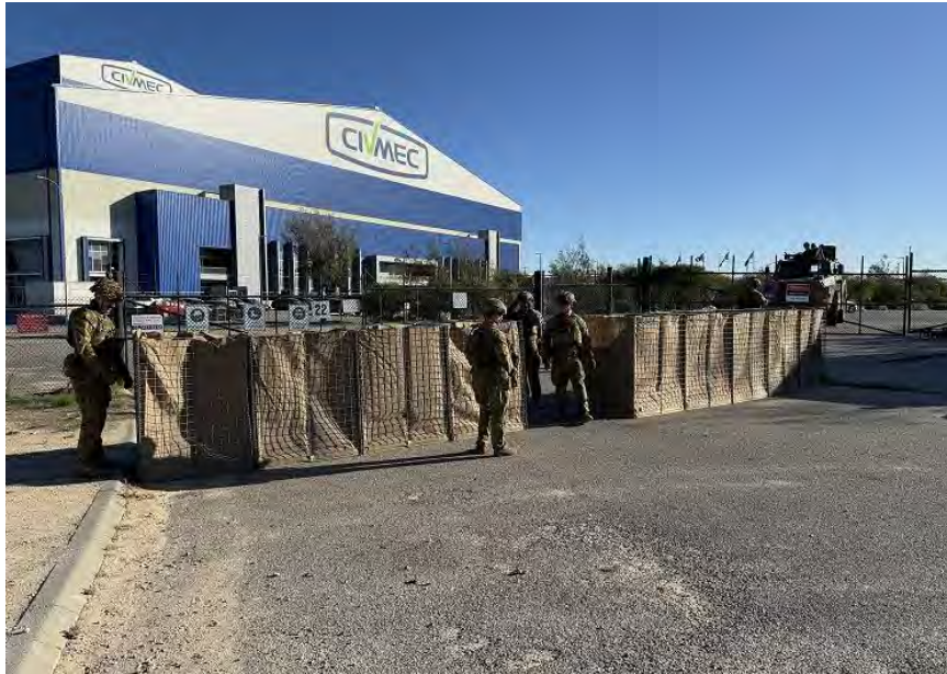
Members of 13 Field Squadron constructing HESCO barriers as part of the wider-area defence plan in support of 16 RWAR at the Henderson Shipbuilding Precinct.
