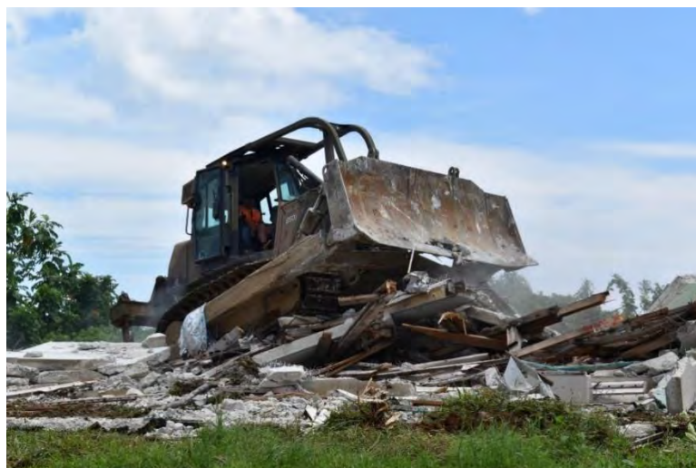
An 850J dozer clearing an old accommodation block at Lombrum Naval Base.
