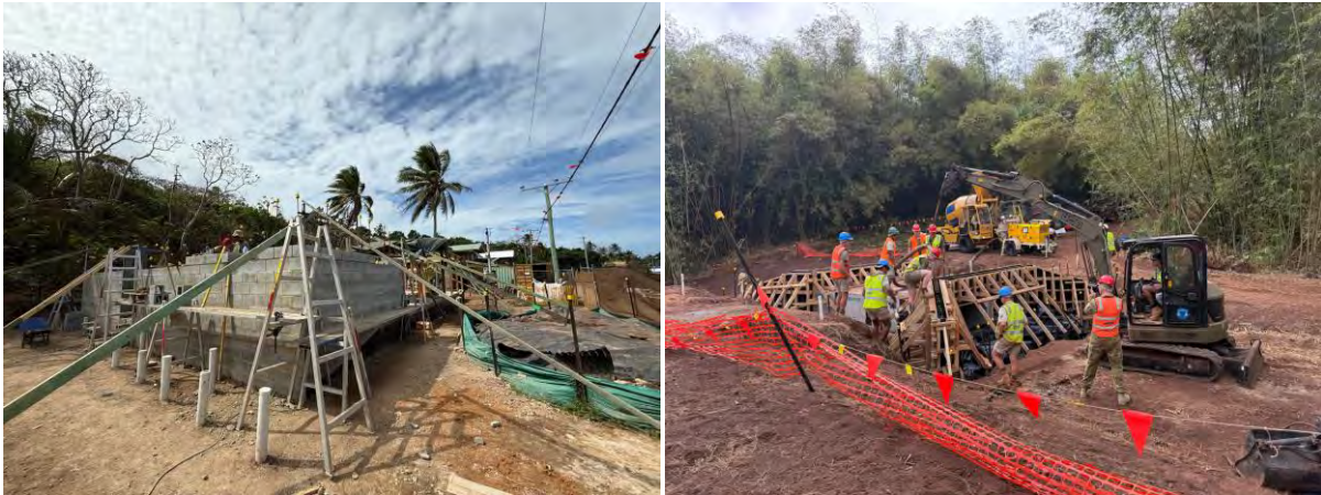
1 TPs Construction of Community Hall (Left) and Concrete Culvert (Right) on Erub.
