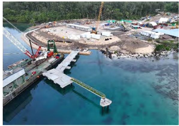
Construction activities in full swing with the first stage of working accommodation and the GCPB wharf emplacement
