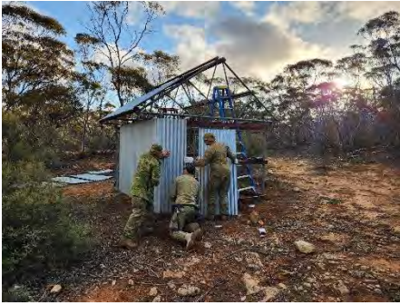
SPR Smith and Construction Troop members SPR Ebert and CPL Malic, clad a hut on EX RHINO RUN 2025
