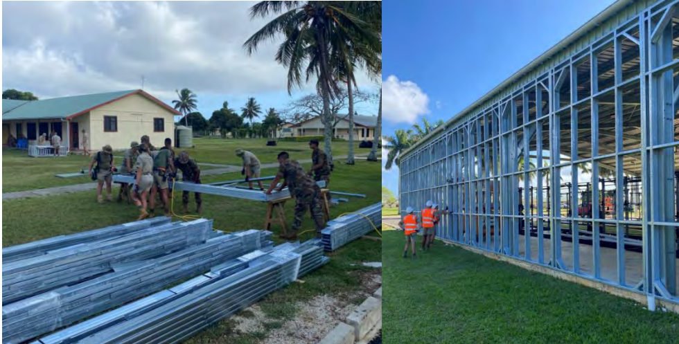
The Exercise Povai Sapper 25 contingent work alongside HMAF engineers building steel frames as part of the gymnasium upgrades.
