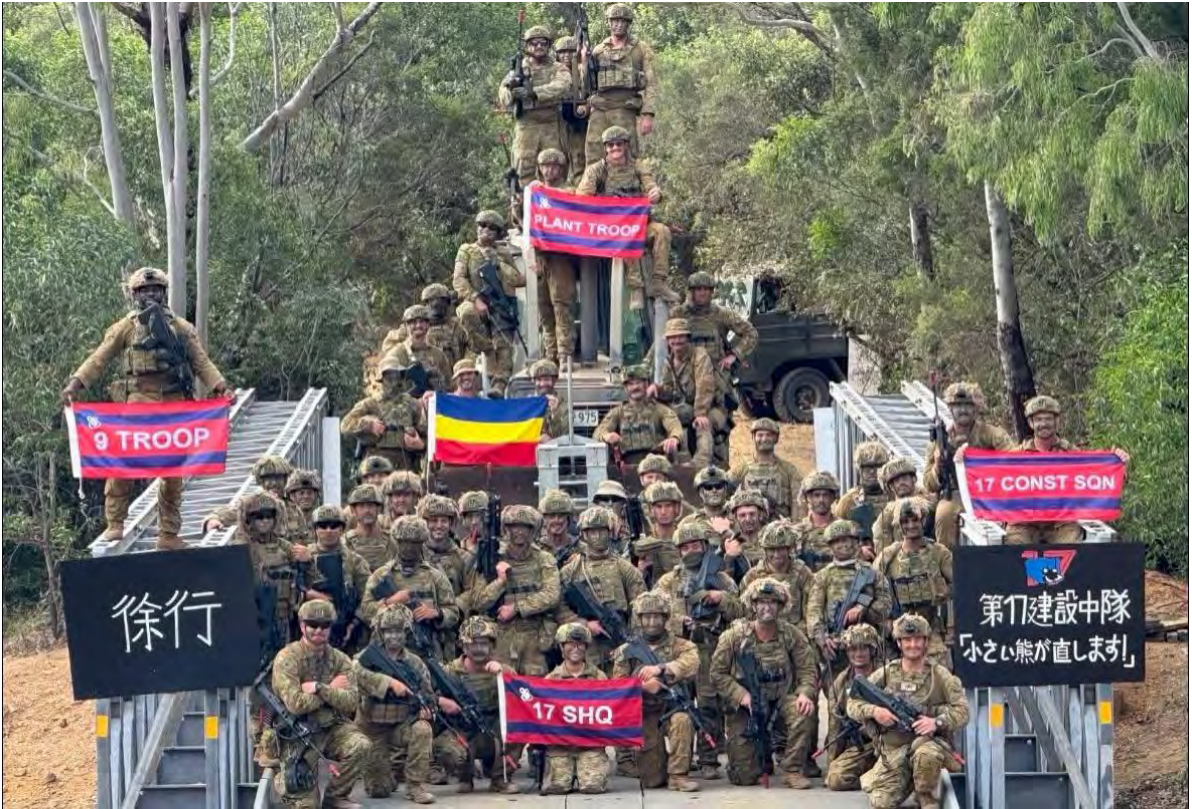
17 Construction Squadrons Fixed Modular Bridge, erected over a wet gap in Townsville on Exercise Brolga Run.
