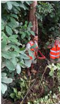
Forward Repair Team (FRT) in action during AACAP 25, delivering critical maintenance and keeping the mission moving in the Torres Strait.
