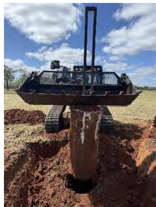
Pozi-track SSL installing a Windsock at Macrossan Airfield, Townsville as part of Ex Global Dexterity 25.
