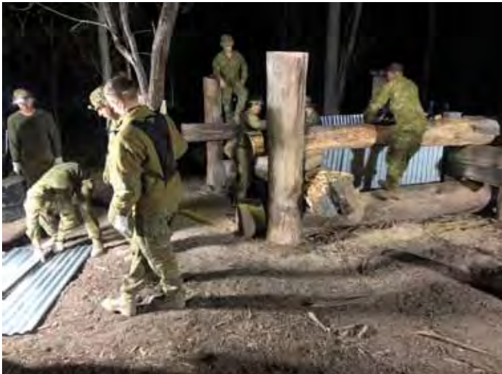
Above: 11 CES Sappers working through the night to complete a log crib obstacle during Ex Rapid Repair
