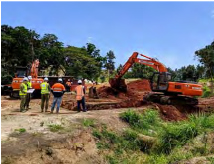
CAPT Mat Jetson, CAPT Gerard Koen, WO1 Pete Gardiner, inspecting earth works conducted by and local contractors as part of the Blackrock Camp Project, Fiji.
