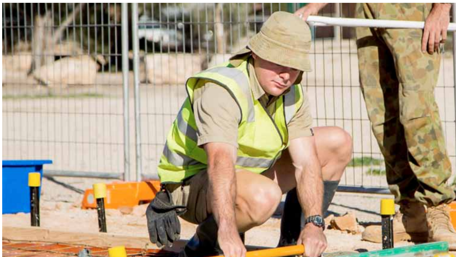
Above: SPR Dayman from Resources Troop screeding the new footpath that now provides access to the local medical facility.
