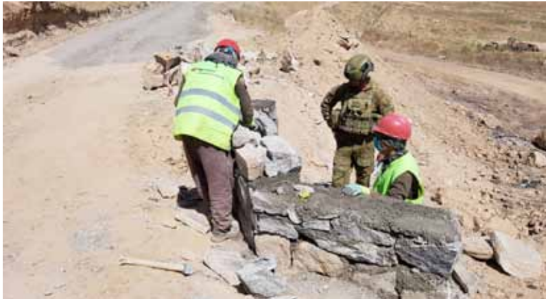
WO2 Coady conducts an inspection of drainage works as part of the road remediation works at Field Marshal Fahin National Defence University, CTA.
